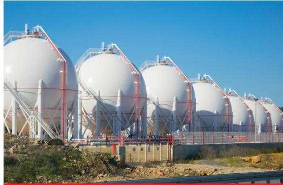
Figure 11: KPC Bulk LPG Storage Handling
