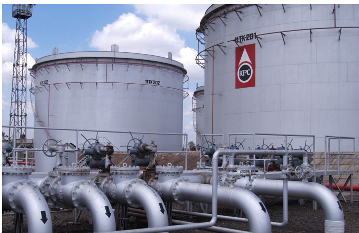
Figure 1: KPC pipeline Storage Facilities
