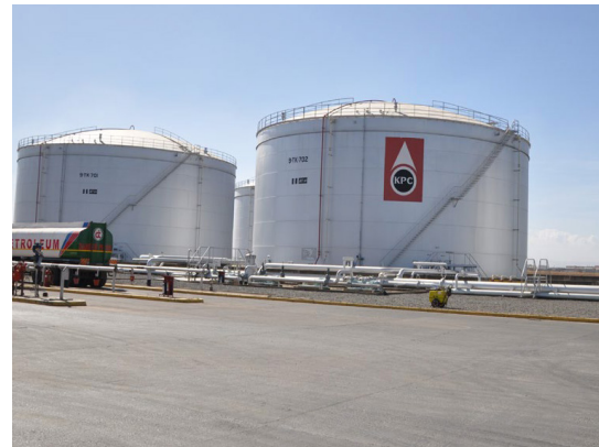
Figure 4: Nairobi Terminal Tank Farm
