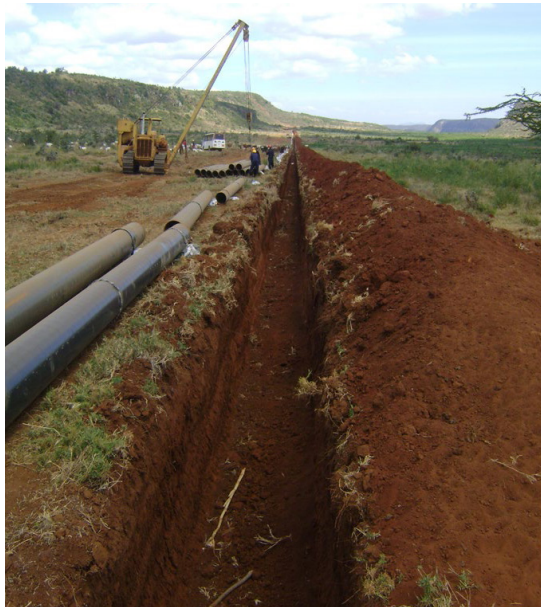
Figure 3: Construction of a 450KM pipeline from Mombasa to Nairobi (Line 5) commissioned in 2018
